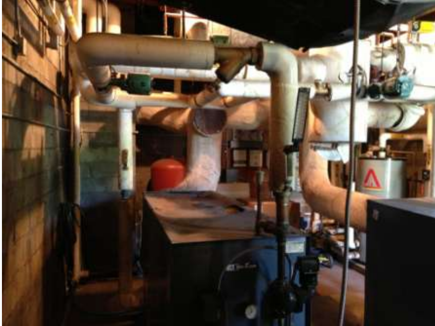
Figure 2. Interior of Lyme School Boiler Room
